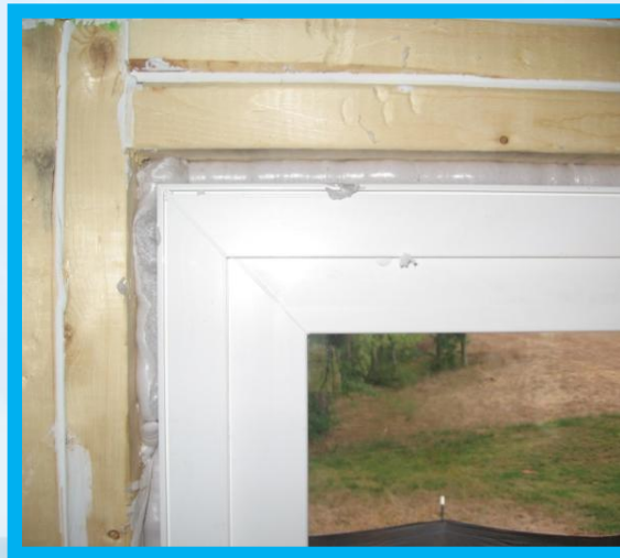
Seal around windows
